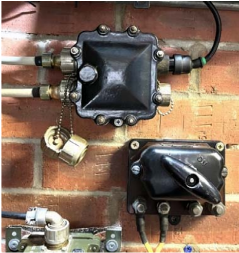
Figure 30. The induction loop box showing the two (12-core) cable ends of the loop entering the box on the left hand side via the Plessey Mk 4 brass connectors, and the connection back to the 5 W amplifier from the right hand side via the Belling Lee push-fit connector. Also note the (original) battery master on-off switch at the bottom right
