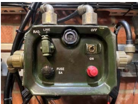
Figure 24. The radio-line box
