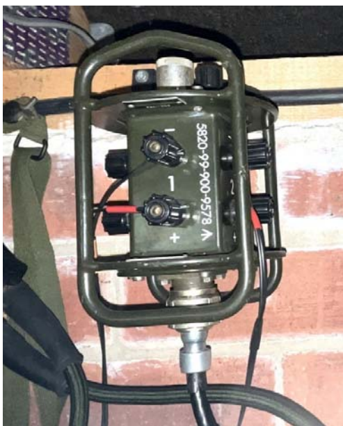
Figure 16. One of the two interconnecting box, terminal units
