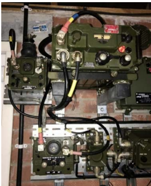
Figure 12. The B48 (mounted on its carrier type 81) complete with its ATU No. 10 and VHF rejector connected into the system. Note the VHF antenna base on top of the ATU
