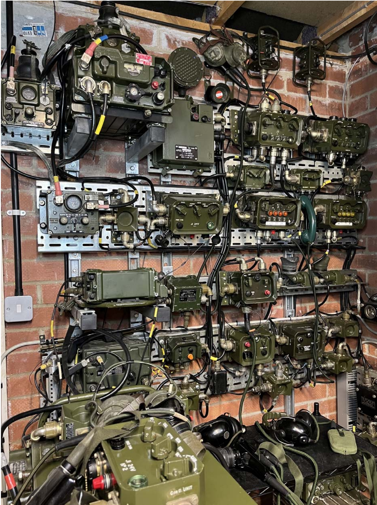
Figure 34. The completed Abbot and command post installation (excluding the driver's section, shown in Figure 26). The command post's C45 A-set and its associated items are at the bottom left corner
