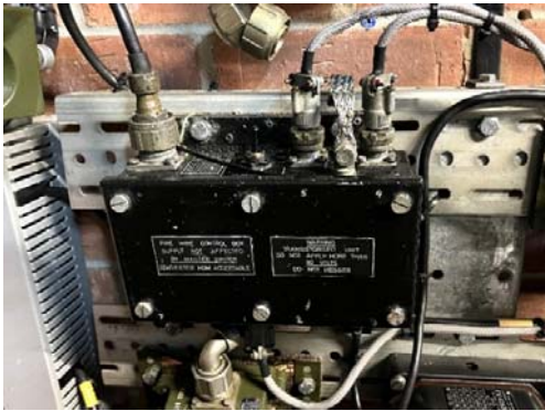
Figure 32. The Graviner firewire control unit. The firewire connections enter via the two Thorn connectors on the top right of the unit
